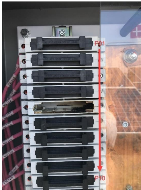
Figure 10 30A fuse holders showing where solar circuits combine into a string, P05 burned out
