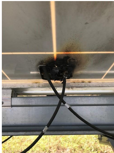
Figure 12 Failed solar panel connection
