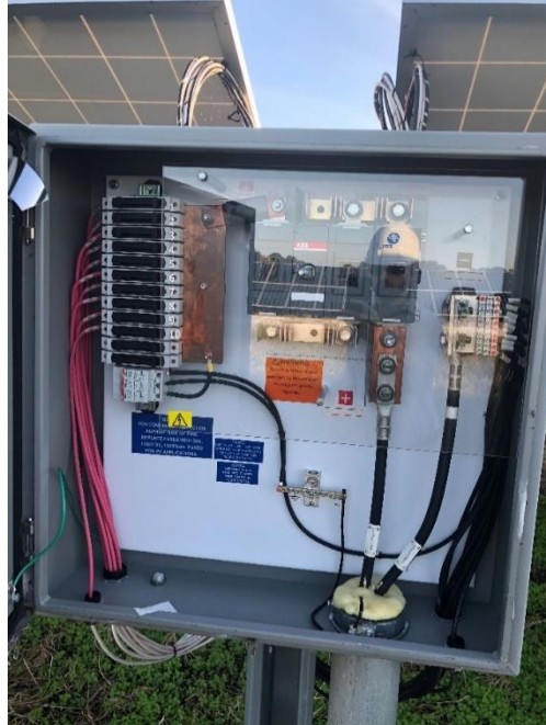
Figure 9 Inside a combiner box, showing solar circuits coming in tied to a 30A fuse
