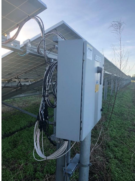
Figure 8 Combiner box where solar panel circuits meet to form a string
