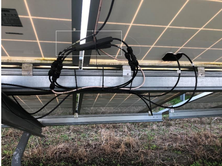
Figure 11 In-line fuses located directly under solar panels, both defective
