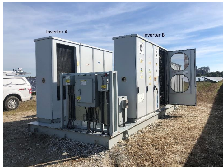
Figure 1 An Inverter Skid
